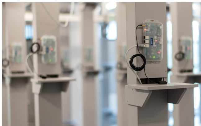
IoT sensors at the French Node - Credit: Inria Photo G. Scagnelli.
